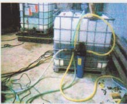
Tank of 1 m 3 volume with a solution IFT-D and mechanic filter 5 microns
